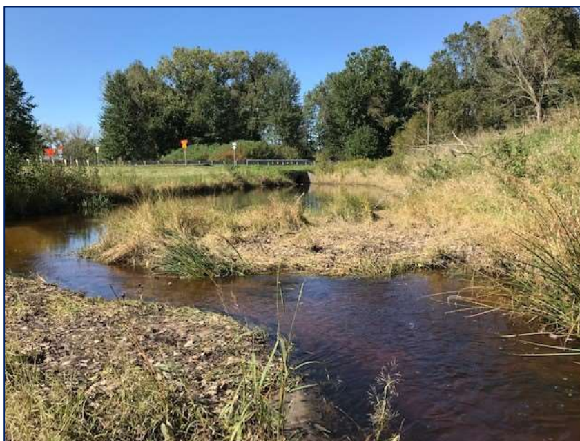
Figure 20- In-line detention basin adjacent to M-140. Photo taken on October 7, 2019.
