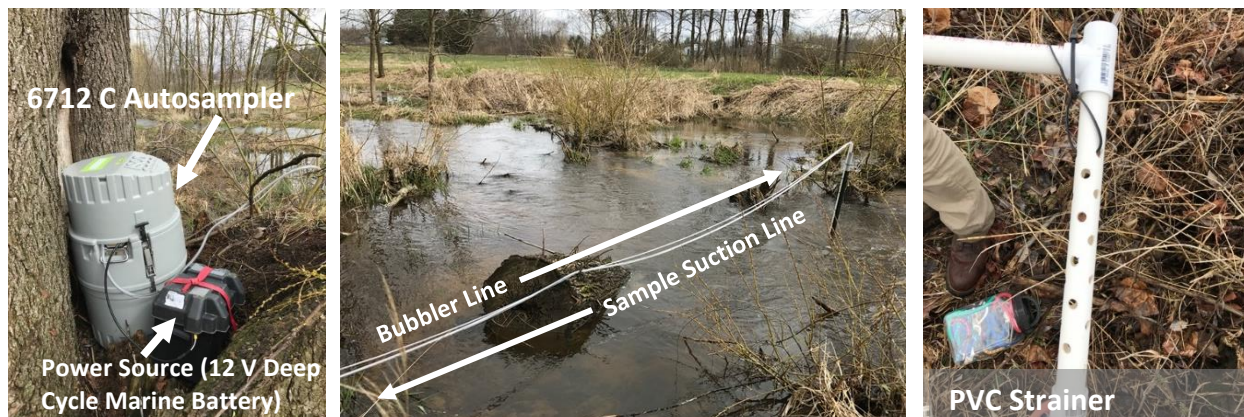
Figure 5 - Field installation of an autosampler on the Branch & Derby Drain (sample site A6). The autosampler is placed on an elevated, flat area, is connected to a power source (12 V deep cycle marine battery), suction line, and bubbler line. The suction and bubbler lines are installed in the drain's centerline and are encapsulated within the PVC strainer. The strainer ensures that when samples are collected through the suction line, nothing large like leaves, crayfish, etc. get stuck in the tubing. Similarly, the strainer protects the bubbler line from damage and a clogged line.
